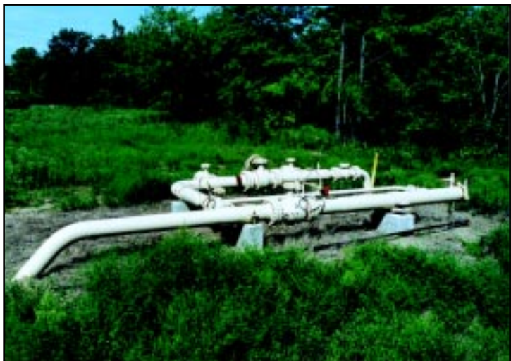
Fig. 6: Natural gas pipeline in southeastern Oklahoma.
